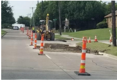
Construction Companies Group (CCG) is continuing to work on panel replacements on Rowlett Rd. between Miller Rd. and Dogwood Trail.
