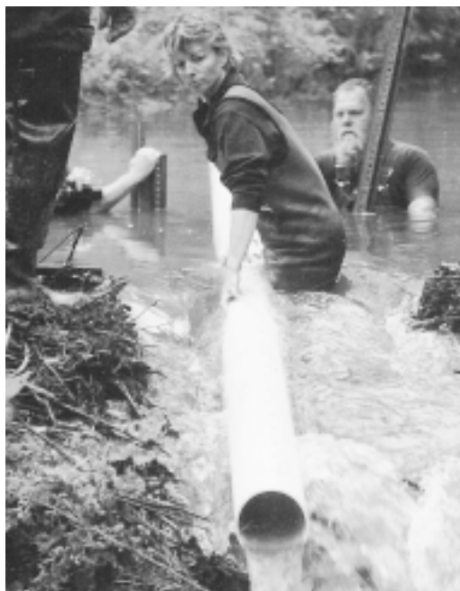
PVC pipes can be run through beaver dams to control flooding problems and to deceive beavers who don't realize that their dam has been breached. Above, Deb Gode installing pipes with the Army Corps of Engineers in Tennessee.
